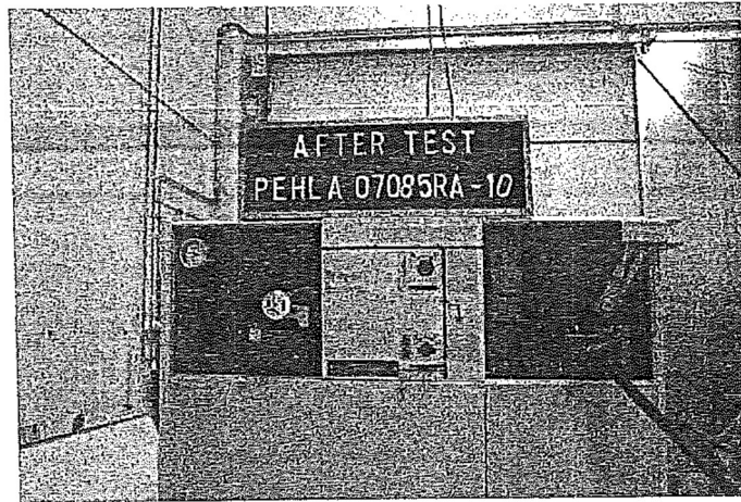
Photo No. 07 After test PEHLA 07085Ra / 10
