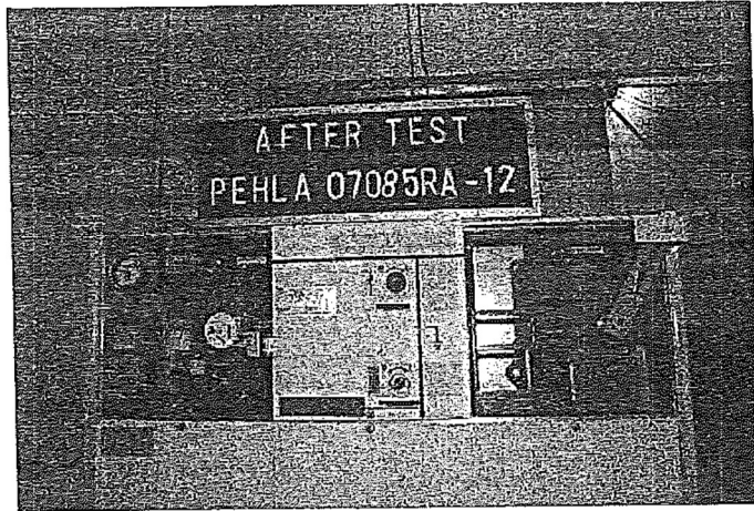
Photo No. 11 After test PEHLA 07085Ra / 12
